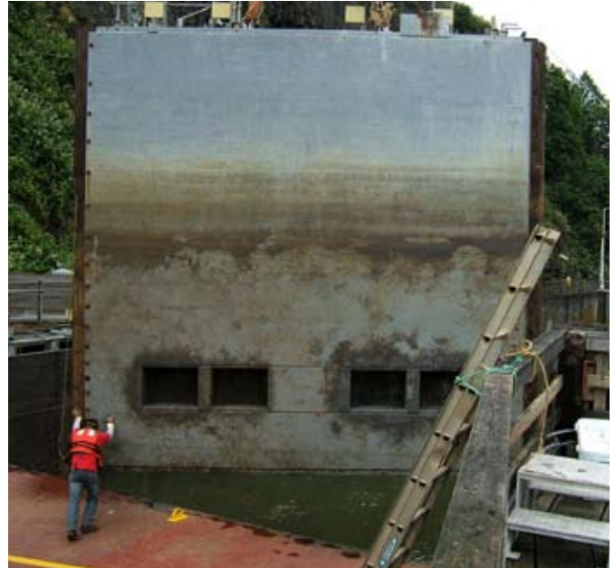
June 15 saw the reinstallation of Gate 7, at the upriver entrance to the canal.
