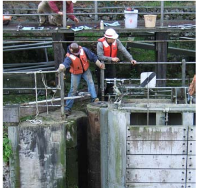
As a leaf of Gate 1 hung from huge straps, workmen resorted to pushing the quoin timber with their feet to protect the shore-mounted fittings during removal.
