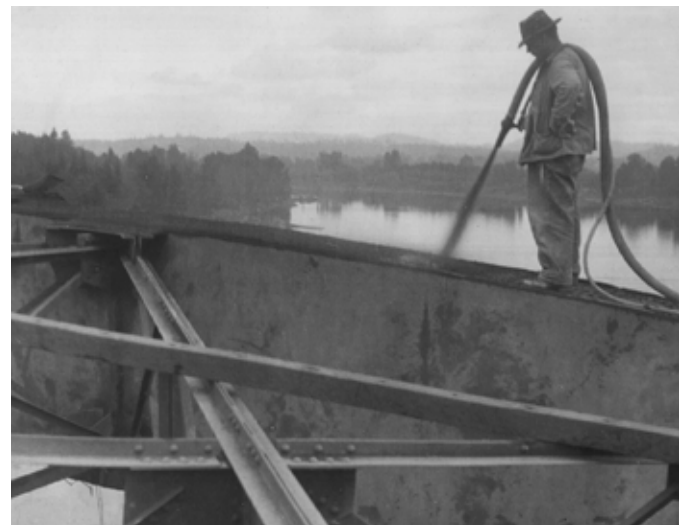
Looking north, this ODOT file photo shows a worker spraying Gunite on the top of the arch during final phase of the 1922 Oregon City bridge construction. Photo from ODOT collection.
