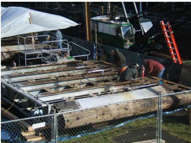
Lock Gate 3 rests in the park February 11 as the crane that pulled it from its hinges awaits its next ‘lift’, back into position after repairs are done.
